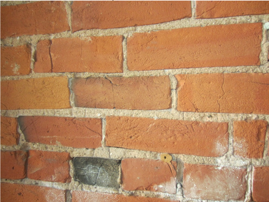
Photo #8: Visible cracks
