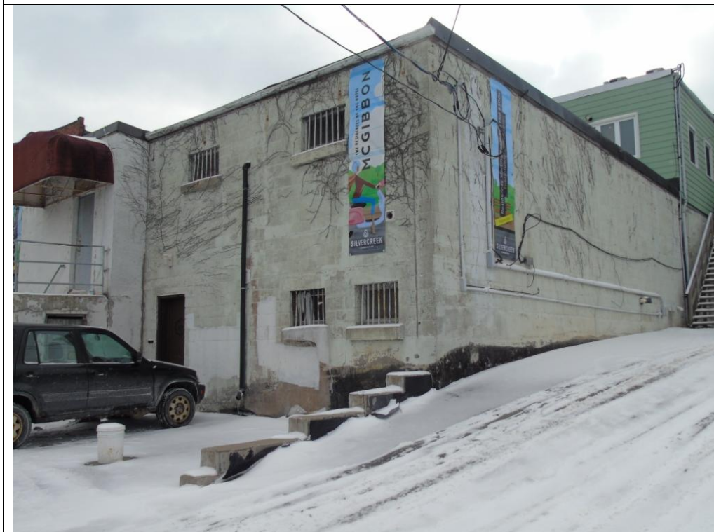
Plate 6: East and north elevations of the concrete block addition at 69 Main Street South, looking southwest.
