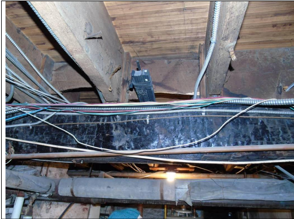
Plate 73: Basement of 79 Main Street South, showing charred hewn wooden support beam, damaged by 1880s hotel fire.
