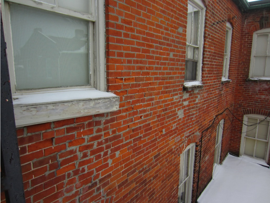
Photo #7: Visible cracks and repair on facade
