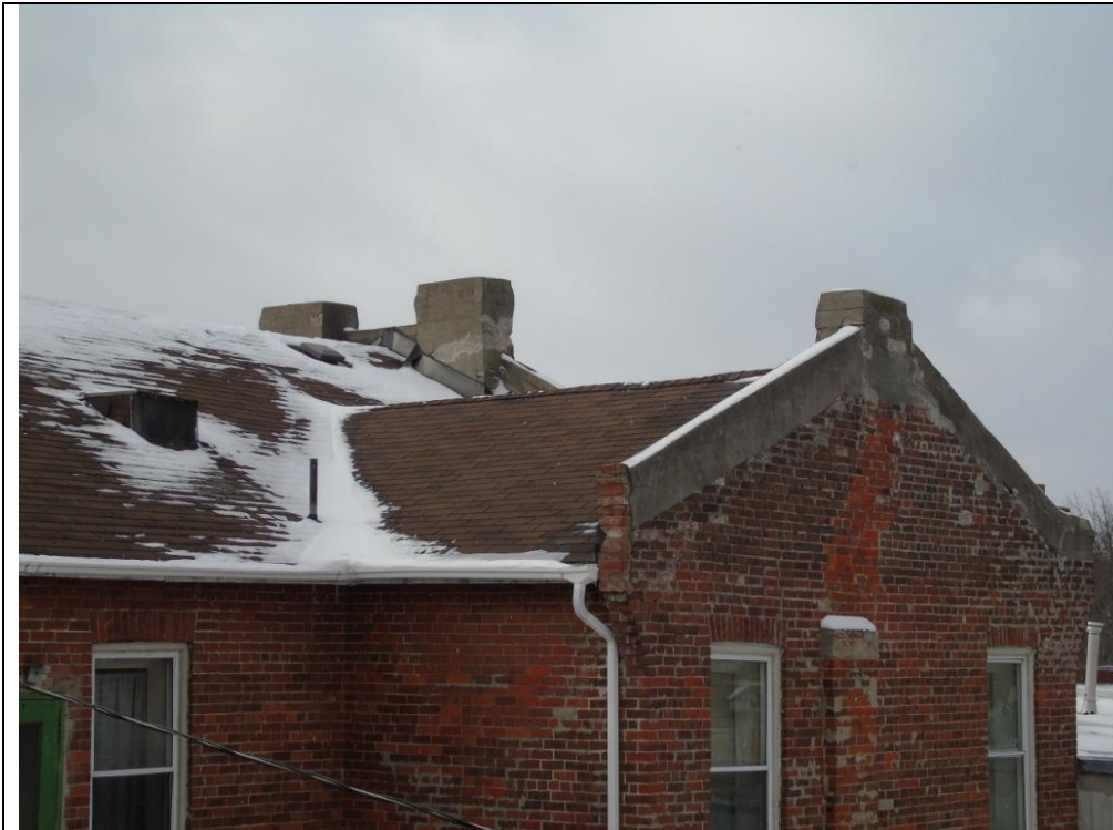
Plate 35: East elevation of 71-77 Main Street South showing intersecting gable roof and parapet, looking northwest.
