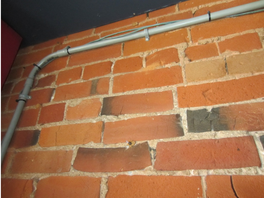
Photo #9: Visible cracks
