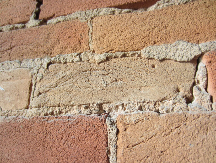
Photo #11: Visible cracks
