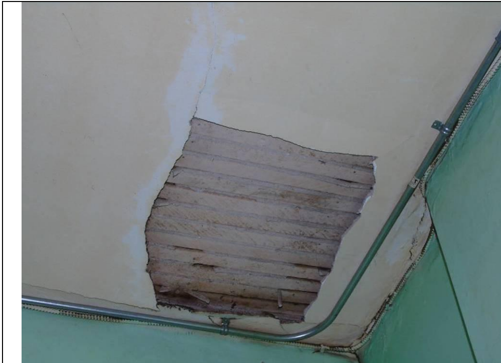
Plate 57: Original lathe-and-plaster was found throughout.
