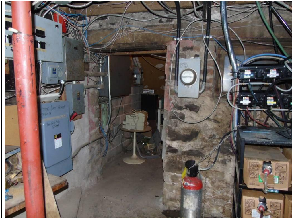
Plate 65: Basement of 79 Main Street South, showing stone foundations, hewn beams, and modern electrical panels.
