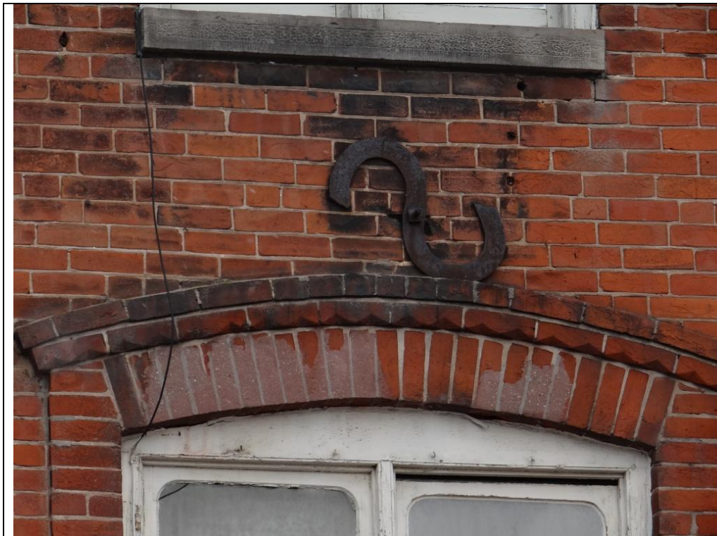
Plate 45: West elevation of 79 Main Street South, showing segmental arches on the window and decorative metal tie-ends, looking east.
