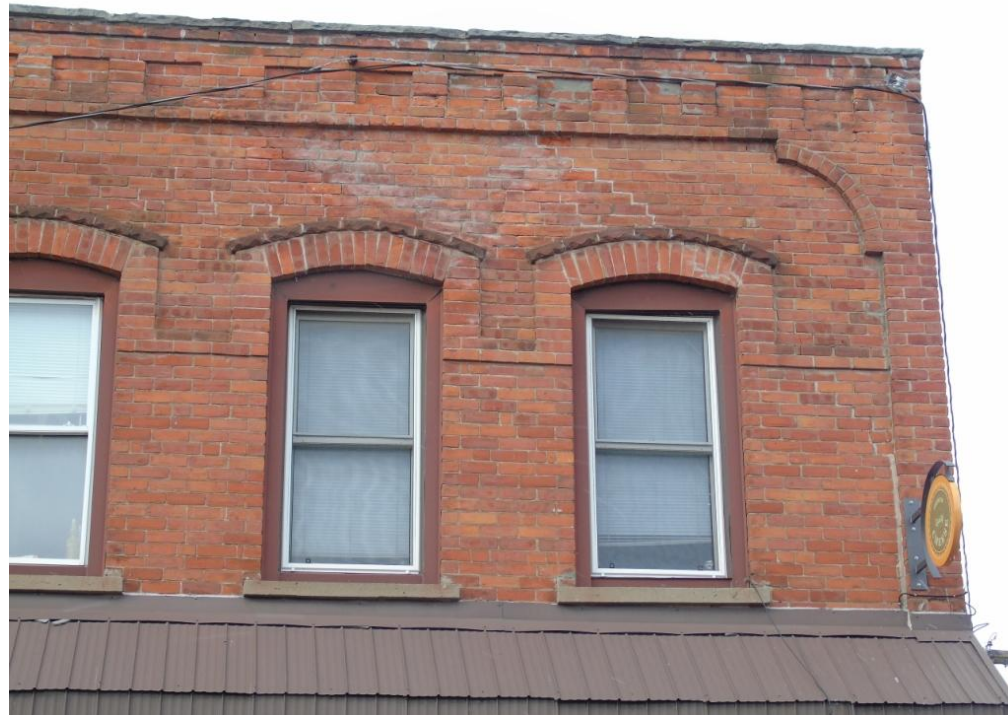
Plate 18: Details of the second floor fenestration and decorative brickwork on the south elevation of the structure at 94-96 Mill Street, looking north.
