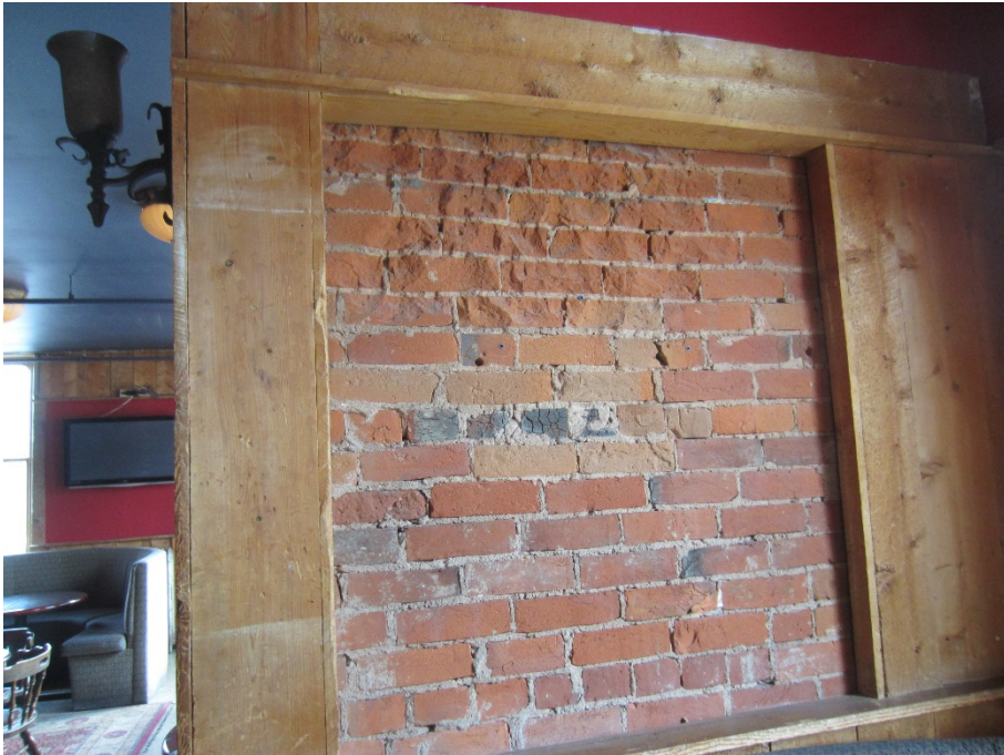
Photo #10: Visible cracks and spalling
