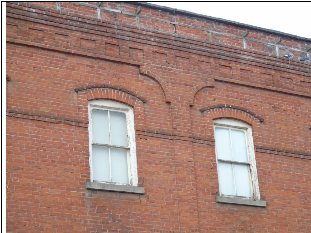
Plate 49: South elevation of 79 Main Street South, showing decorative brickwork, sash windows with segmental arches, and repairs to the roofline, looking northeast.
