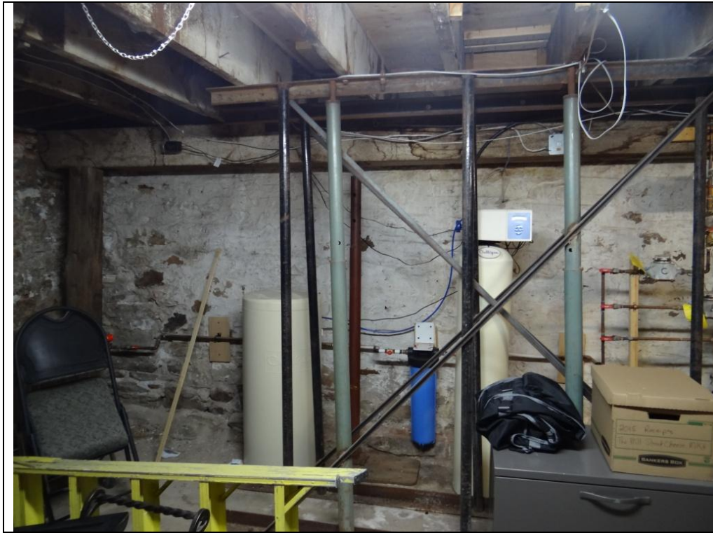
Plate 31: Detail of modern structural steel posts added to reinforce the main floor joists in the basement at 94-96 Mill Street.
