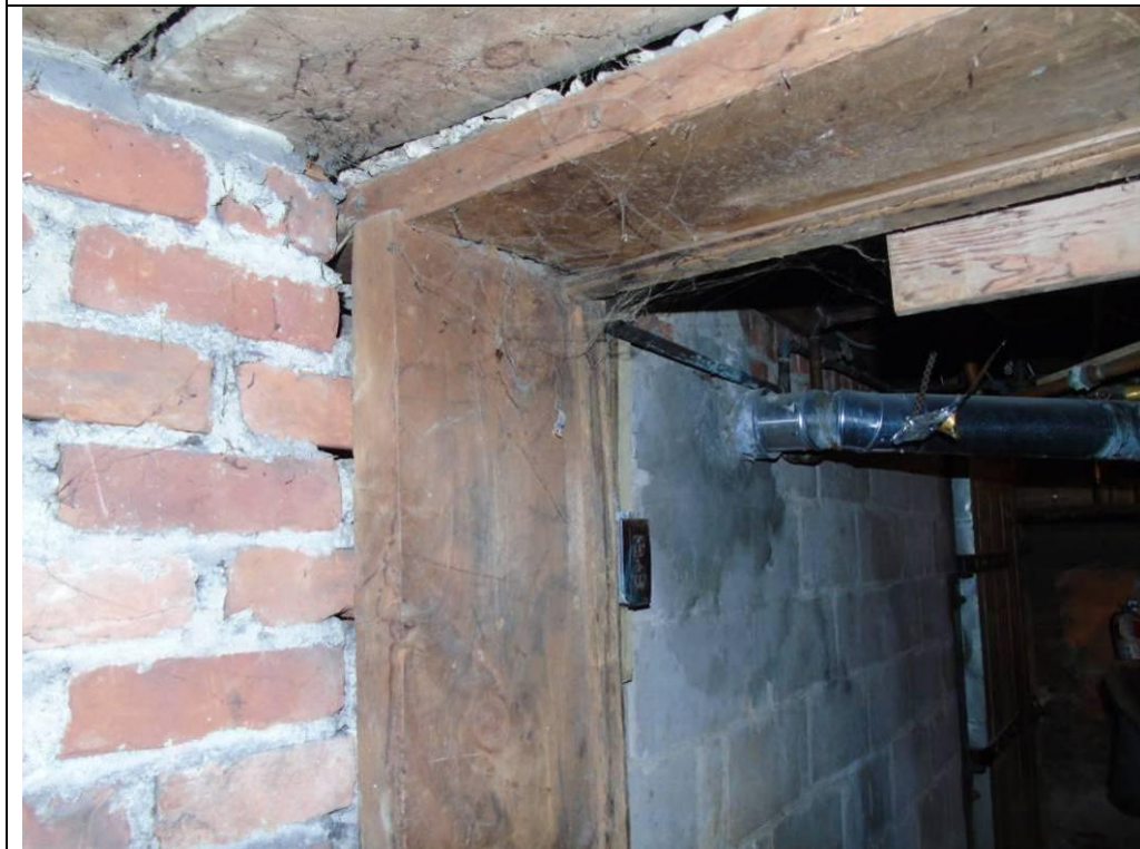
Plate 70: Basement of 71- 77 and 79 Main Street South, showing red brick and cinder block foundations, softwood floorboards, and modern dimensional lumber door framing.
