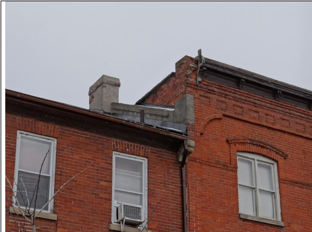
Plate 33: West elevation of 71-77 Main Street South showing stepped parapet separating the structure from attached 79 Main Street South, looking northeast.
