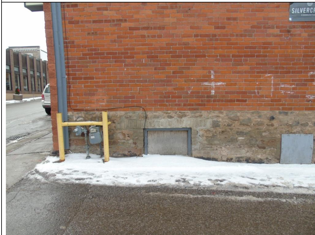
Plate 22: Detail of the brickwork and foundation on the east elevation of the structure at 94-96 Mill Street, looking west.
