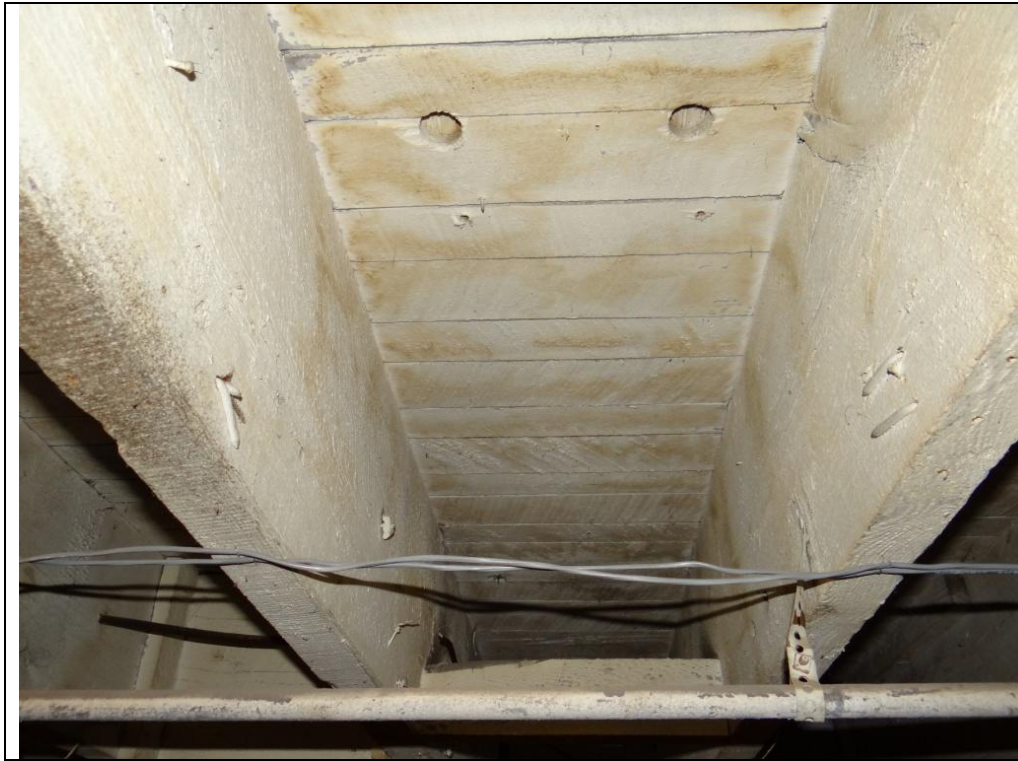
Plate 13: Detail of the sawn floor joists and softwood plank flooring from the basement of 69 Main Street South.
