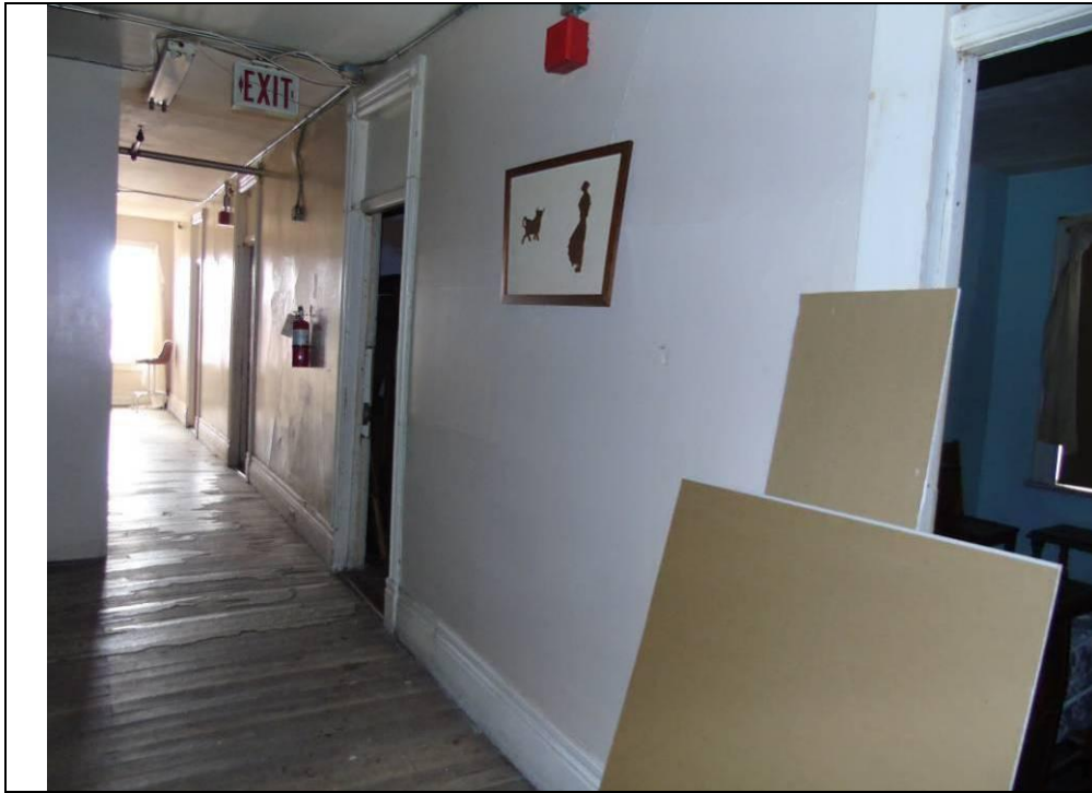
Plate 63: View of the north-south hallway towards the front of the hotel on the third floor.
