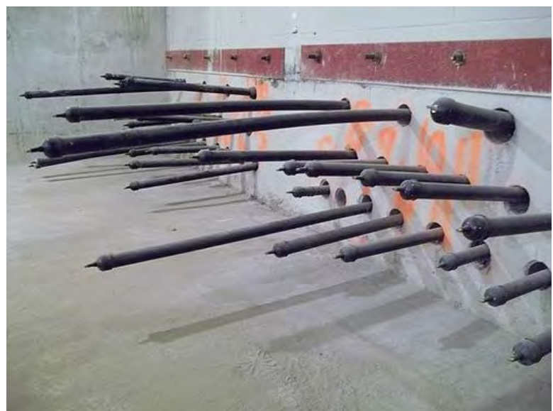
Geothermal piping at the Halton Hills Library and Cultural Centre.
