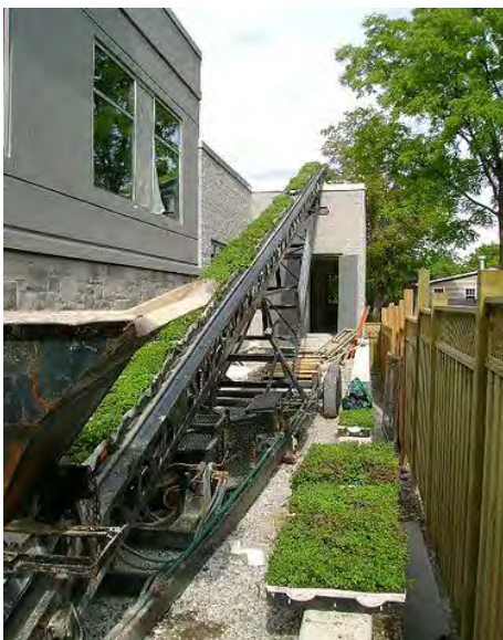
Green roof under construction at the Halton Hills Library and Cultural Centre.
