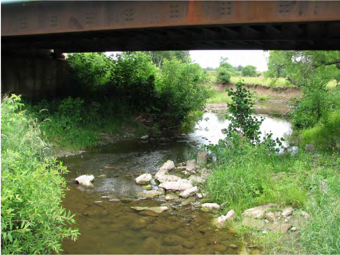
Photo 8: Downstream view to the south of Middle Sixteen Mile Creek Tributary at Station 4. The confluence with Middle Sixteen Mile Creek occurs almost immediately downstream of the railway crossing.
