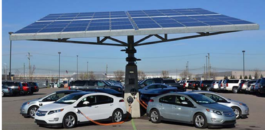
Figure 29 - EV Charging Station
